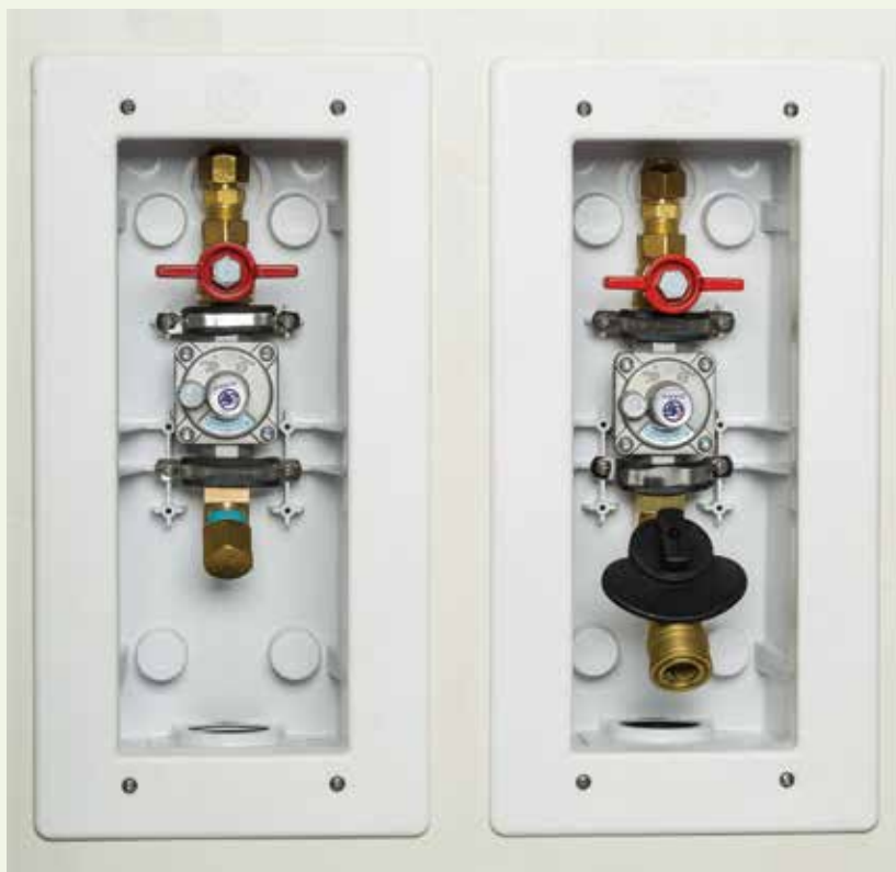
When paired with corrugated stainless-steel tubing, or CSST, convenience outlets (like pictured) provide an easy, plug-in connection to a home's natural gas supply.
